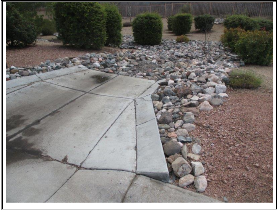
RETENTION BASINS (TYPICAL)
